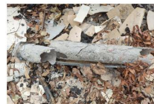
Figure 7 Fire damaged asbestos cement flue.
